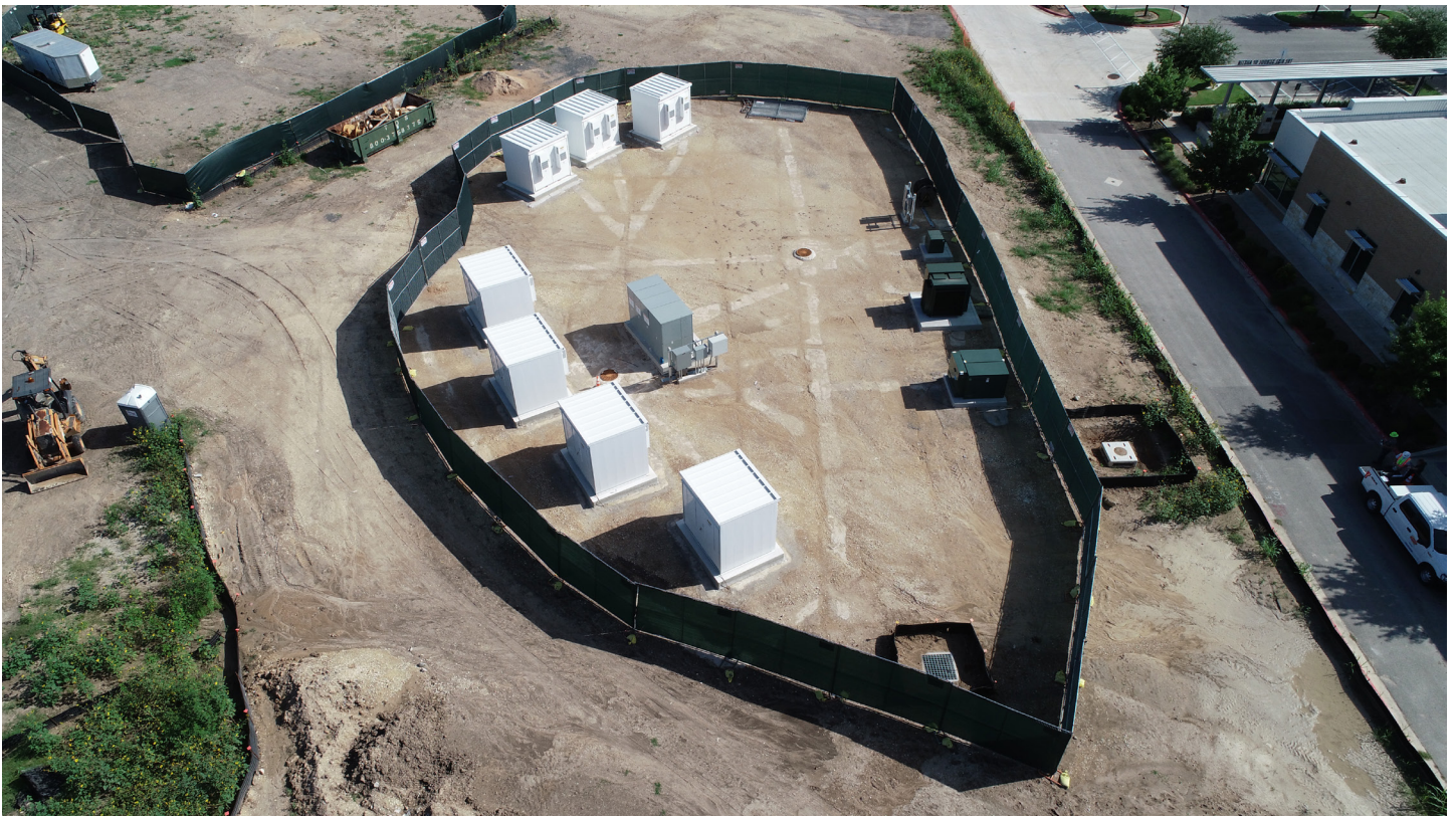
Austin SHINES – Mueller ESS 1.5 MW / 3MWh
