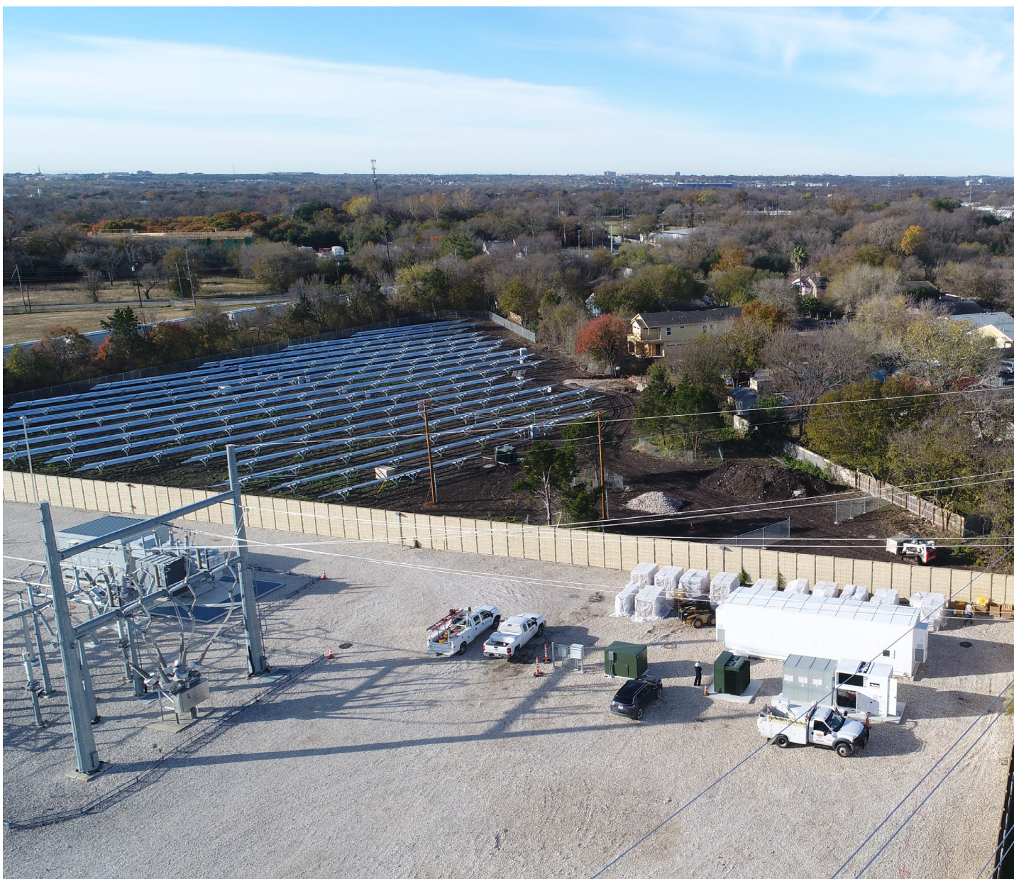
Austin SHINES – Kingsbery ESS 1.5 MW / 3MWh with La Loma Community Solar Farm
