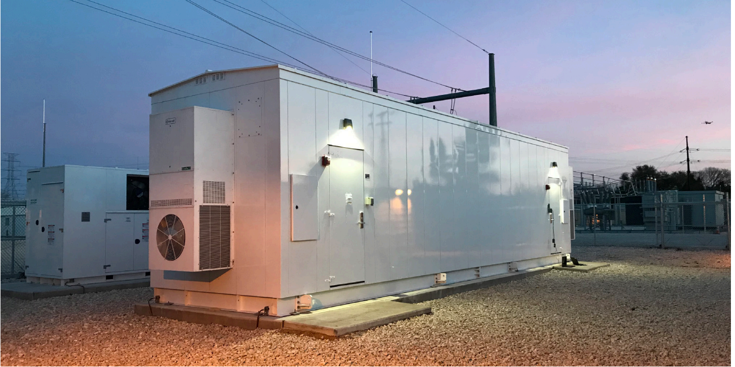
Austin SHINES – Kingsbery ESS 1.5 MW / 3MWh with La Loma Community Solar Farm
